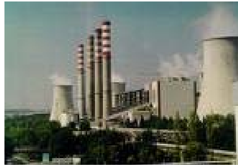
Yona Power Plant (Courtesy of Yona Power)
